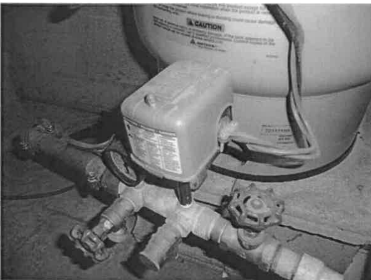
Close-up view of the pressure switch that turns the pump on/off; The blue tank is the pressure tank
