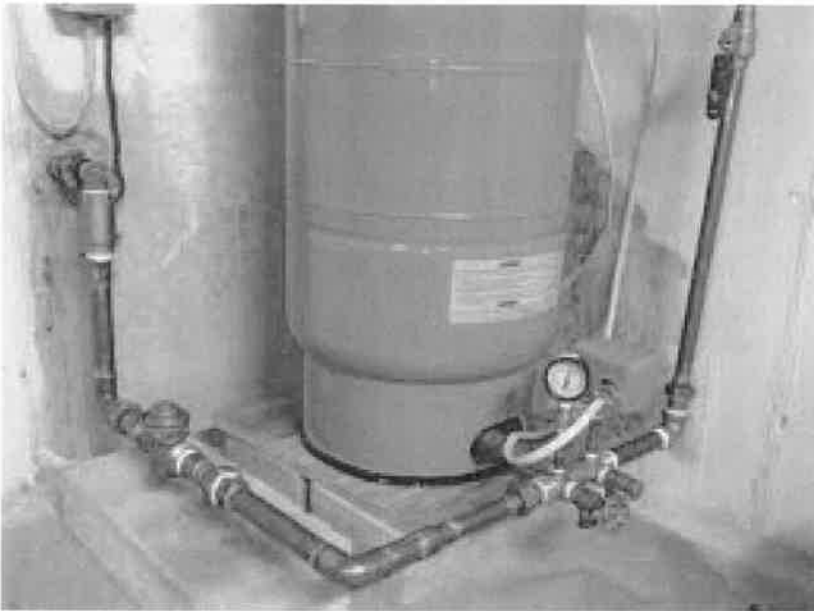
Image of how a well connects to a pressure tank, showing the pressure gauge, pressure switch and storage tank
